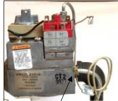
Gas line for pilot.
