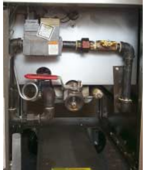
Gas valve in the MJ35.
